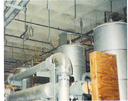
San Andreas Water Treatment Plant San Francisco, California Engineer: Camp Dresser & McKee
